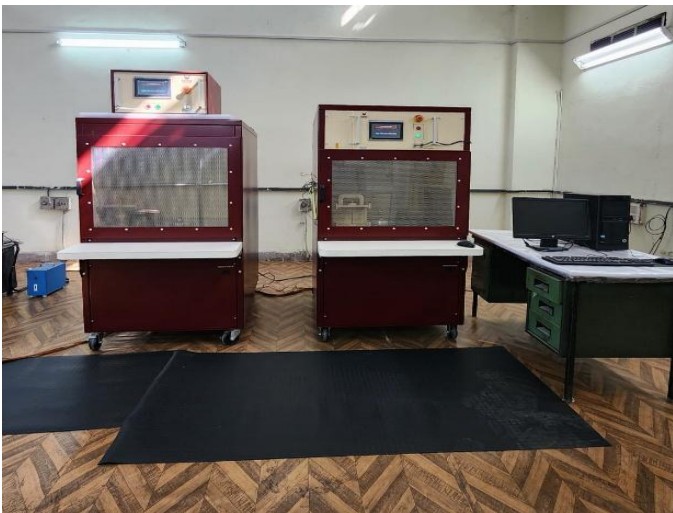
AC DC HV TEST SYSTEM
